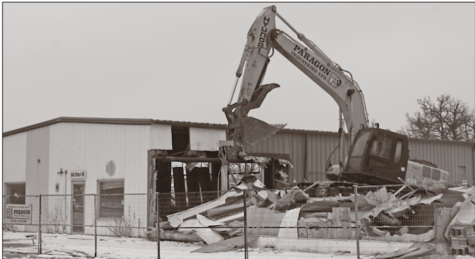
The old CANEX building gets torn down to make way for new development. Photo: Mike Sherby
