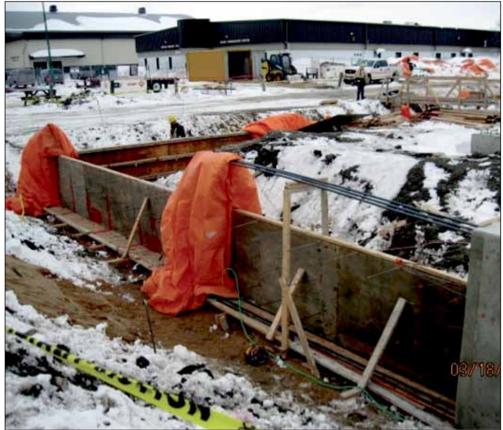
Construction in progress at the new CANEX building in March 2014. Photo: Supplied
