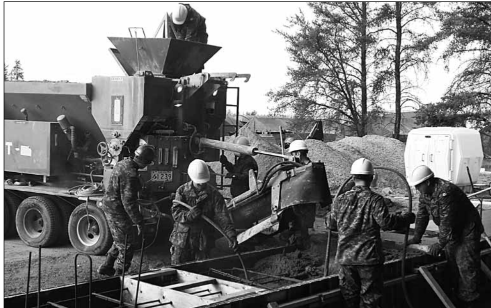
17 Wing personnel make and place concrete, using the volumetric concrete mixer, for the front footing of a storage building. Photo: Submitted
