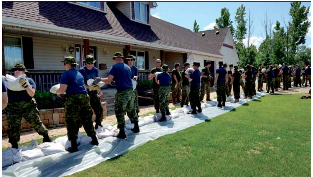
Canadian Armed Forces members from 17 Wing, Winnipeg and CFB Shilo help move sand bags in preparation for flooding across the Manitoba region in support of Op Lentus, just outside St. Francois Xavier, July 8, 2014. Photo: Cpl Paul Shapka
