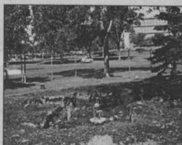
The future site of the CF 104 on the Left Hand side of the gate.
