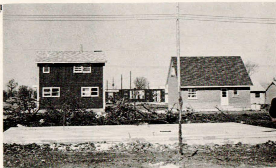
Situated behind one of the slab foundations are a number of Metropolitan Construction Co.'s new PMQ units in various stages of near completion at the new PMQ development.
